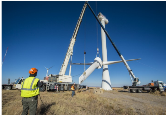
Engineers changing rotor blades on a wind turbine (c) Dennis Schroeder / NREL CC BY-NC-ND 2.0
